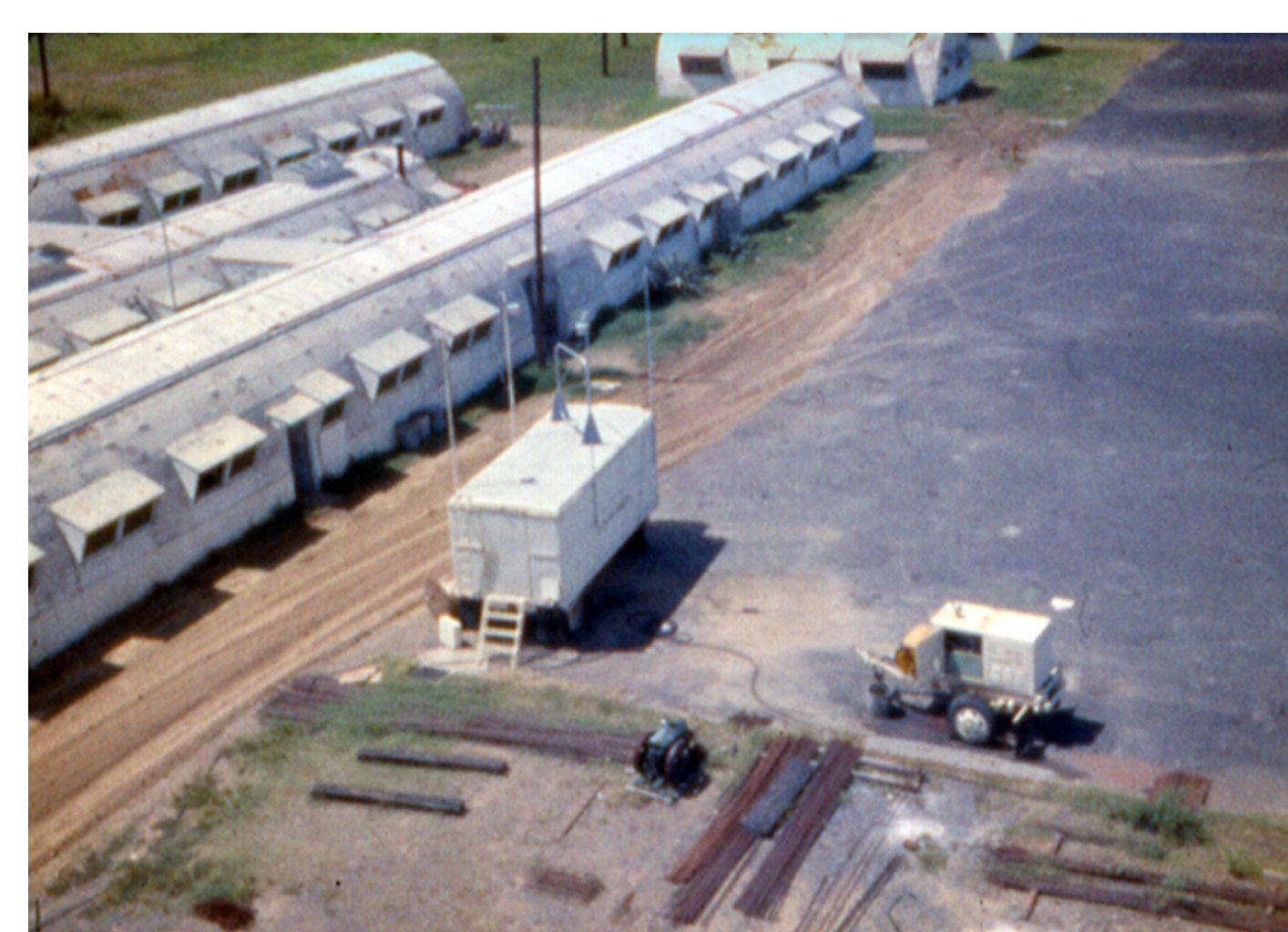
Doppler Shift satellite tracking van showing the tracking antennas, the Loran-C antenna, diesel generator, and housing.
